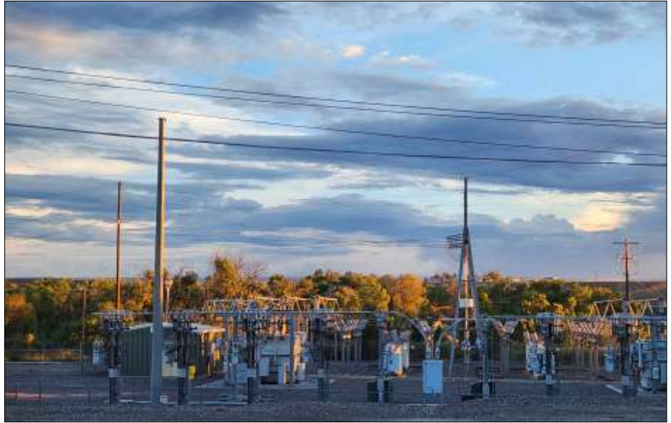
On the night of July 26, the Delta Montrose Electric Association (DMEA) Bullock Plant substation lost power for a couple of hours. Chief Executive Office Jack Johnston reported the event during the board of directors during the July 28 regular board meeting. Johnston said, "It was a curious racoon. At 11:45 p.m. half the power was knocked out. The racoon was fried. Curiosity killed the racoon!" Mirror staff photo.
