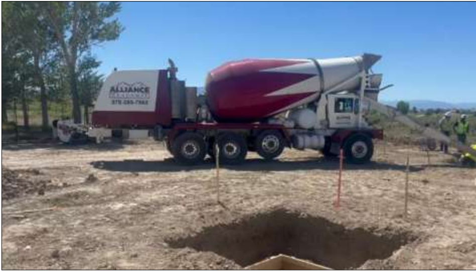
Alliance Ready Mix pouring concrete at the new Montrose Veterans Memorial site June 17, 2026. Photo by J. Bob Brueske.
