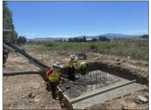
Double A workers finishing the concrete in the forms at the Montrose Veterans Memorial site June 17, 2026. Photo by J. Bob Brueske.
