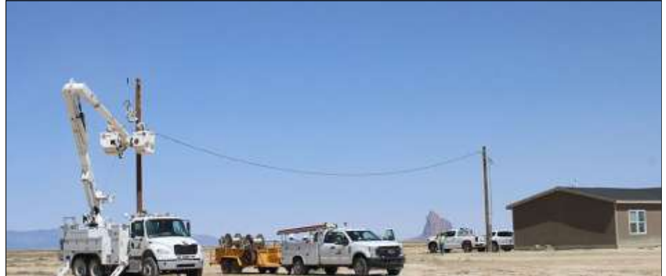
Delta-Montrose Electric Association (DMEA) line crews recently returned from the Navajo Nation after participating in the Light Up Navajo initiative DMEA courtesy photo.
