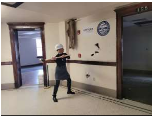
On Monday, Feb. 5, Montrose County held the Golden Sledgehammer Ceremony which commemorated the start of renovations to the Historic County Courthouse. Following opening remarks from officials, Montrose County Commissioner Sue Hansen was given the honor of striking the first demolition blow. Still, damage to the sheetrock wall to the left of the electrical outlet was less than impressive. BOCC Chair Roger Rash said, "Sue, you hit the stud!" After other participants helped Hansen's first attempt at demolition look more respectable, she was determined to leave her own mark. She said, "Let me try it again!" Photo by Gail Marvel.
